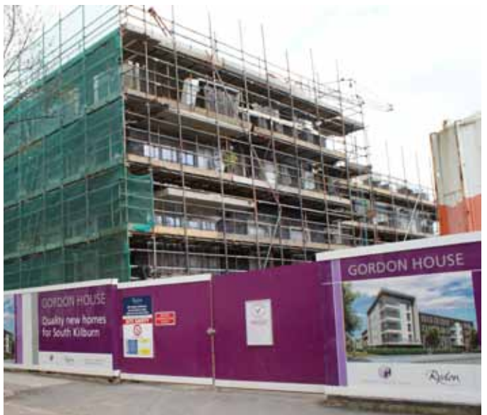
Network Housing and Rydon Homes are making progress where Gordon House used to be. McDonald House will contain 26 new homes for social rent, including family-sized units with private gardens and terraces
