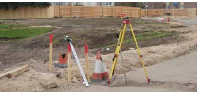
Removing the Carlton Vale roundabout has created a sizeable space which is being prepared by London & Quadrant for building to blocks containing 133 new homes
